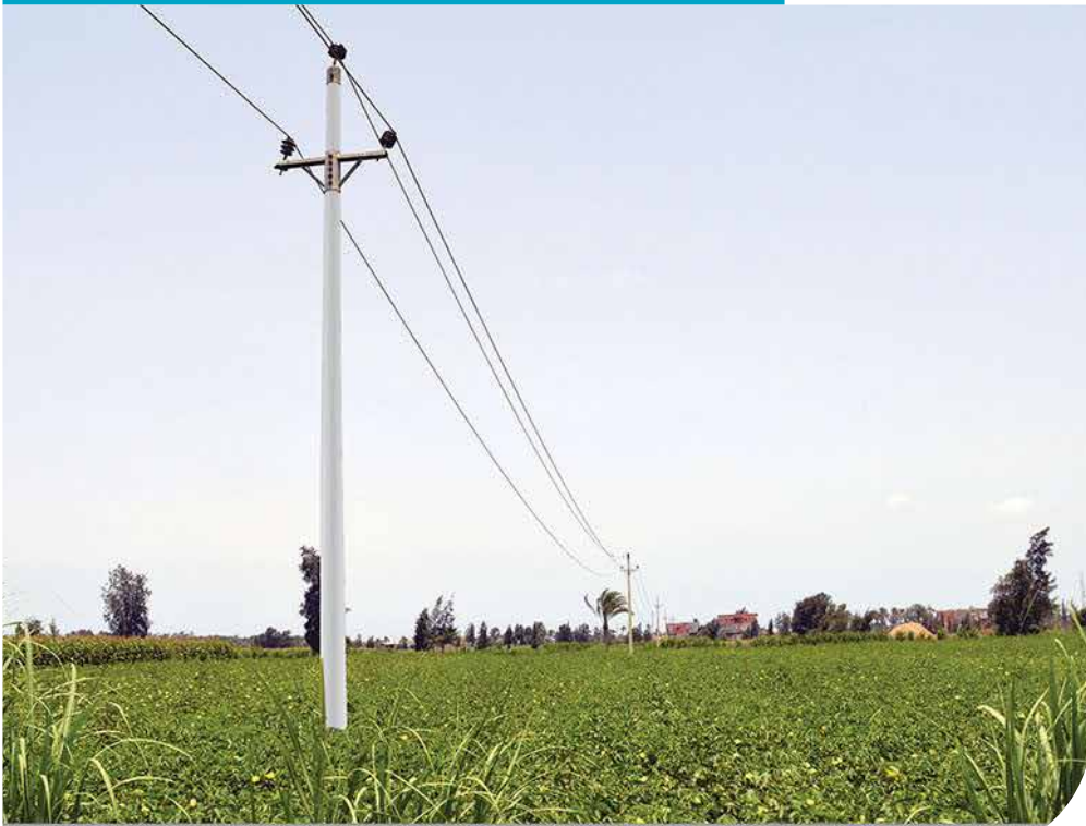
Power Transmission Poles
