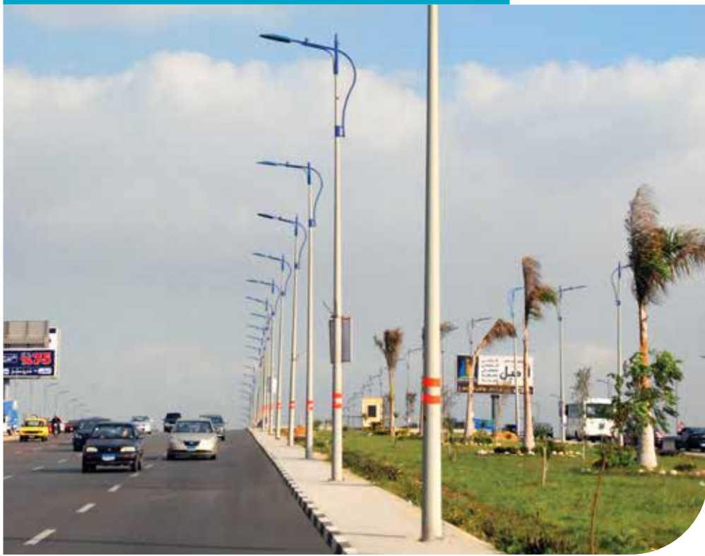
Street Lighting Poles
